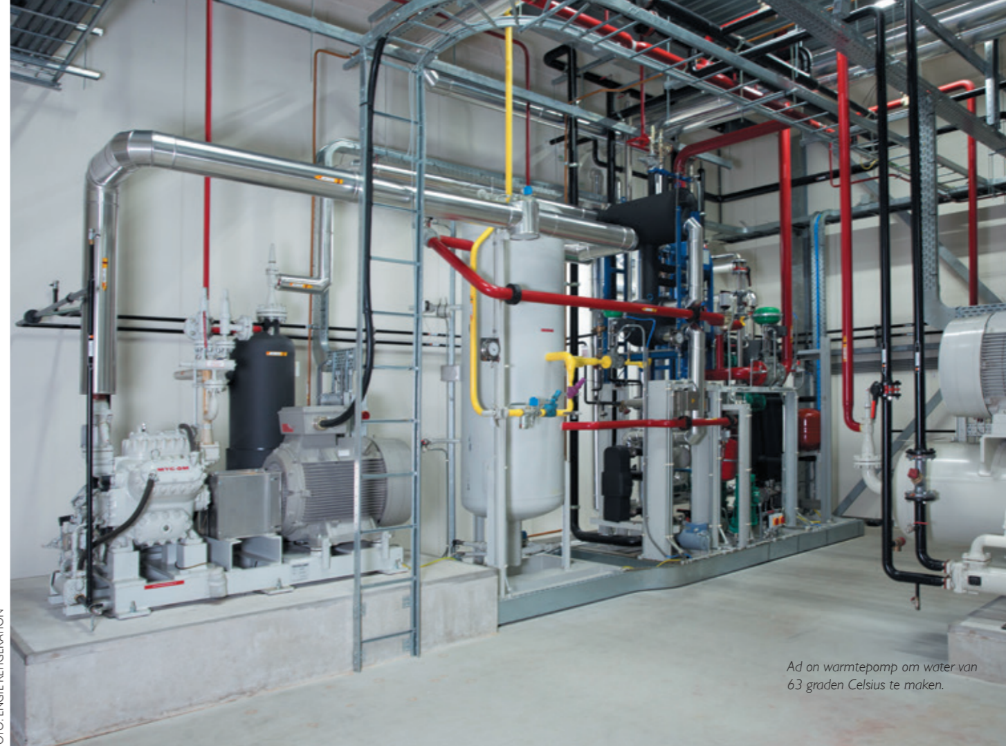
FOTO: ENGIE REFRIGERATION
